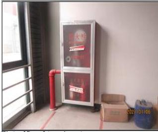
Photo of fire safety equipment 4-3 Fire hydrant.JPG
