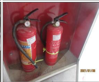
Photo of fire safety equipment 4-1 Fire extinguisher.JPG
