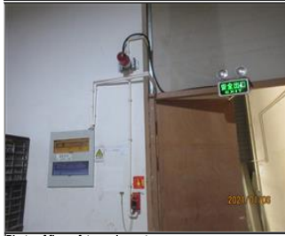
Photo of fire safety equipment 4-2 Fire alarm.JPG
