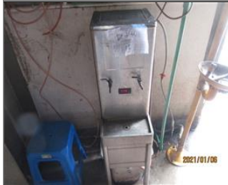
Photo of the sanitary facilities 13-1 Drinking water.JPG
