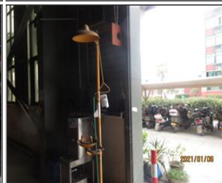
Photo first aid facilities 2-2 Eye washing equipment .JPG
